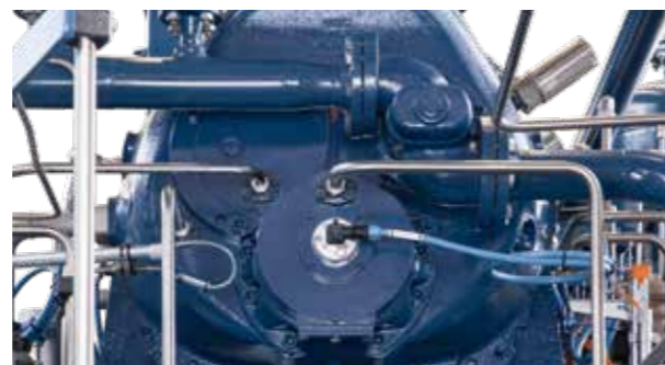
Compressor stage lubrication piping.
